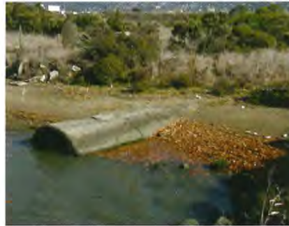
Like many of the creeks around the Bay, Schoolhouse Creek enters the Bay in a storm drain pipe. Photo by Lisa Owens Viani.
