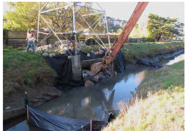
PG&E repair from storm damage in Tam Valley. Credit: Marin DPW
