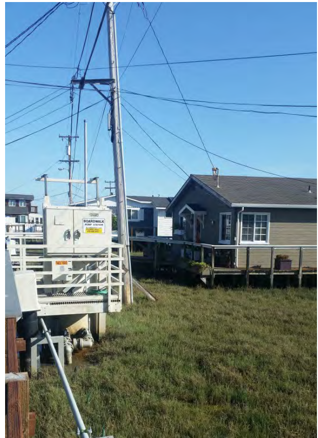
Greenbrae Boardwalk utility lines line the pathway. Credit: BVB Consulting LLC
