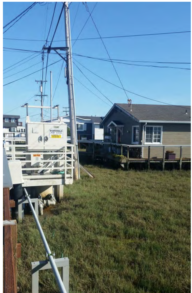
Greenbrae Boardwalk utility lines and control systems. Credit: BVB Consulting LLC
