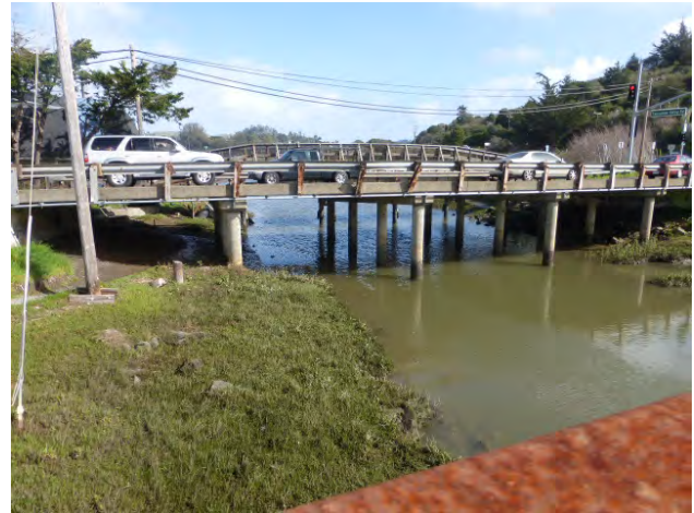
Utility lines crossing Coyote Creek where it enters Richardson's Bay. Credit: Marin DPW
