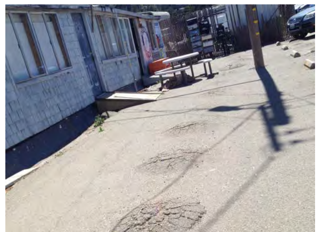
Subsidence in Marinship, Sausalito. Credit: Marin County CDA
