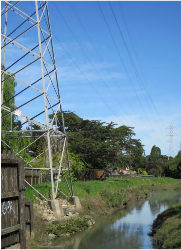
Electric transmission tower on Nyhan Creek levee in Tam Valley. Credit: Marin County DPW
