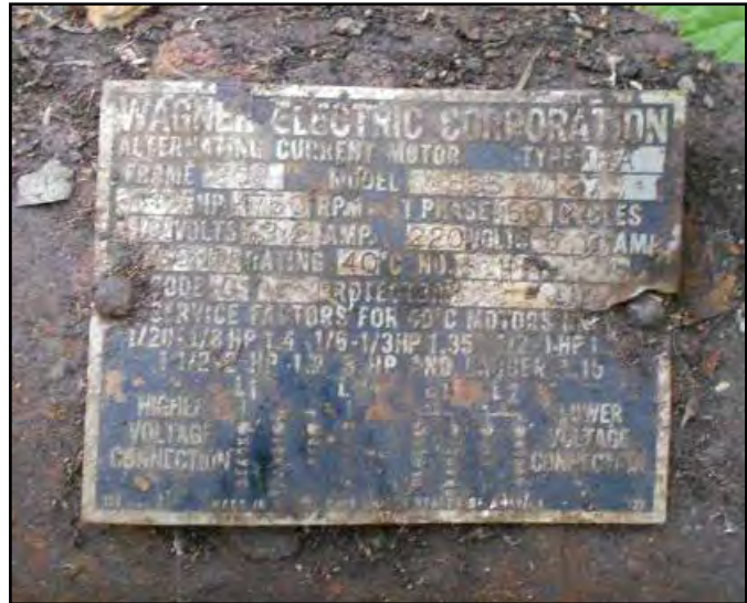
Photo 3. Face plate on pump motor (NorthEnd#2)
