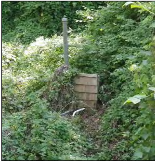
Photo 2. Pump house (NorthEnd#2)
