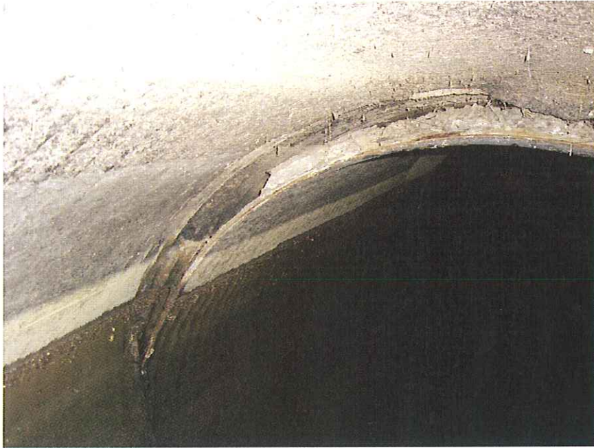
Photo 1 – Deflection at Top of Culvert
