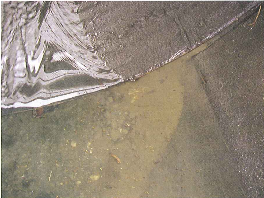
Photo 2 – Settlement at Culvert Invert
