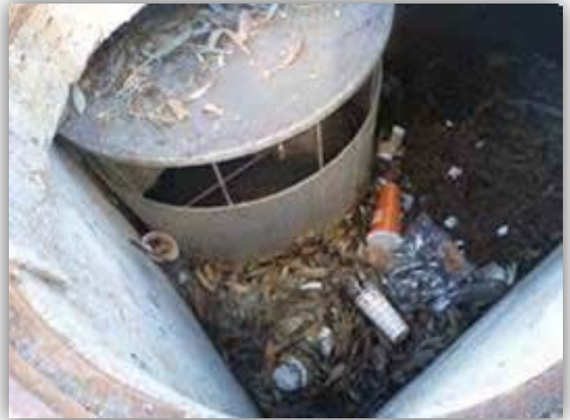
New trash reduction requirements will require Trash Capture Devices in high trash generating areas.
