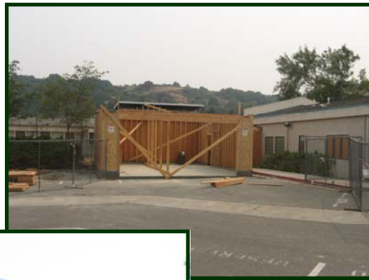
One month into construction on the sally port. Photo taken on June 26, 2008.
