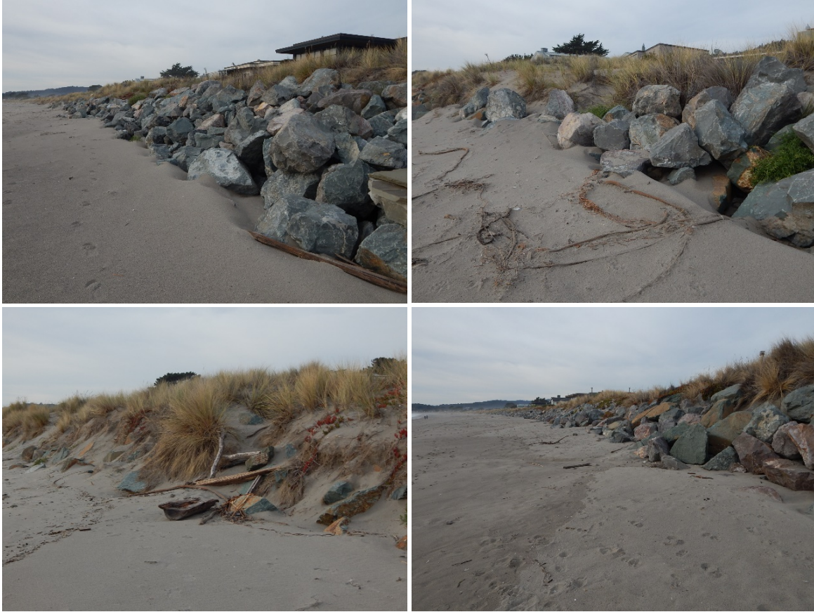
Eastern end of Seadrift rock revetment, December 20, 2019. The boulder revetment here varies between exposed boulders with recent unvegetated wind-deposited sand ramps (SE-oriented) and mixed marram foredunes perched in the revetment, partially eroded or persistent. This profile indicates alternation between severe erosion to the revetment, and episodes of backshore beach and dune accretion. There is currently no significant annual or perennial beach vegetation in the backshore seaward of the revetment. (P. Baye)
