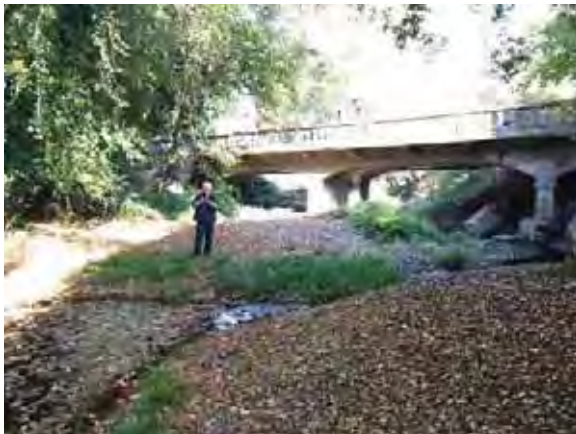
Figure A-8: View of Upstream Face of Nokomis Bridge Notice large gravel bar deposits underneath and in left bay of bridge.
