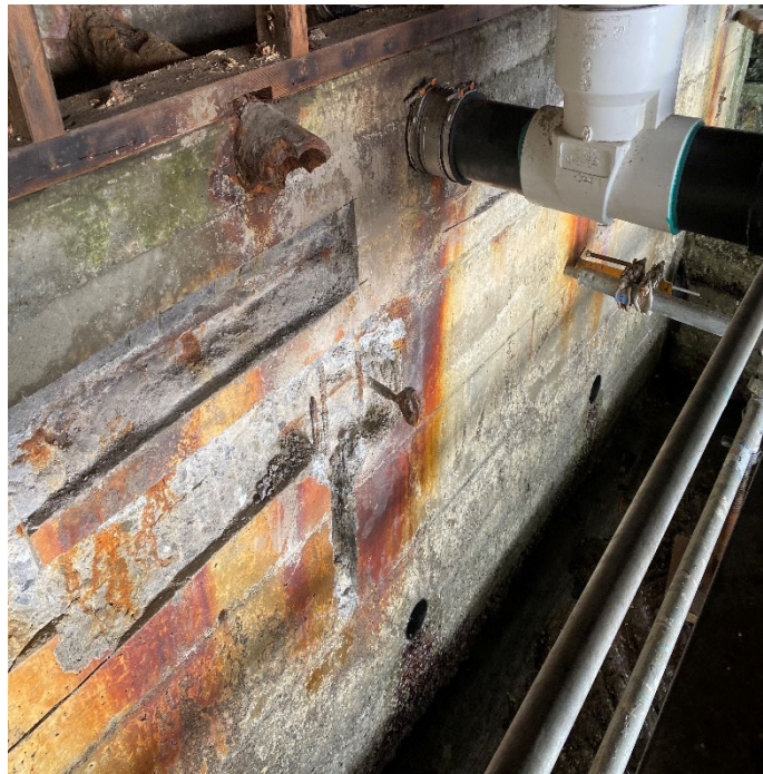
Figure 4 - Reinforced concrete wall showing typical distress, including spalling and exposure/corrosion of rebar.
