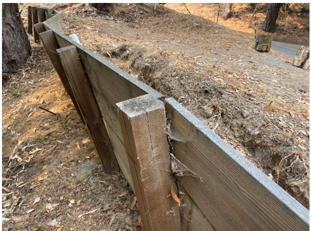
Figure 7 - Typical timber wall with 4x4 posts and 2x12 lagging showing typical distress due to age and rot.
