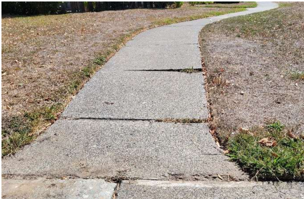
Figure 1. Representative example of sidewalk trip hazards found across the property. Source: MHA, 2022.
