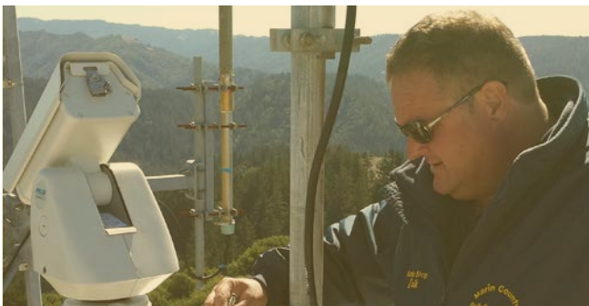
New fire-detection cameras installed on Mount Tamalpais
