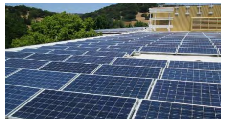
Photovoltaics at 1600 Los Gamos Dr.
