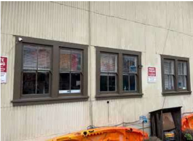
Historic window fabric and placement, January 21, 2024.
