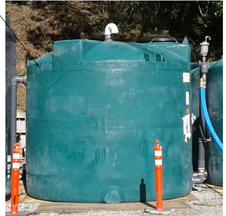
2 6 4,600 GALLON WATER TANK PHOTO SCALE: NTS
