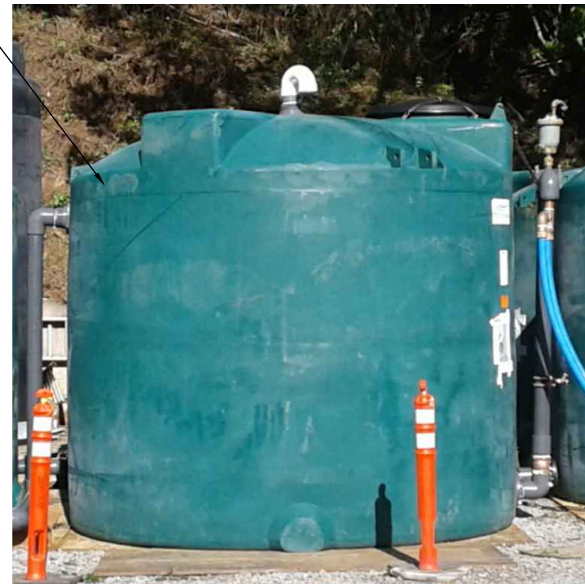
2 6 4,600 GALLON WATER TANK PHOTO SCALE: NTS
