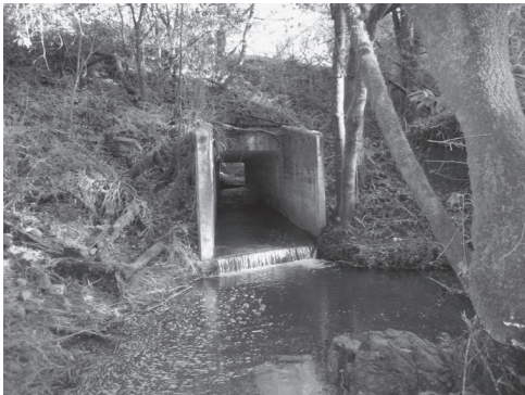
Traditional box culvert with concrete bottom
