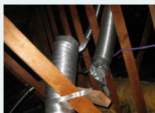
Disconnected Attic Duct
