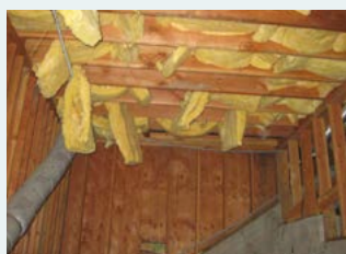
Poorly Insulated Floor/Crawl Space
