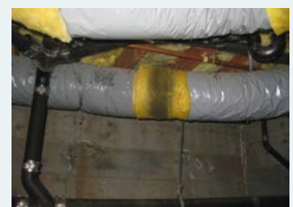
Leaky Duct Seam
