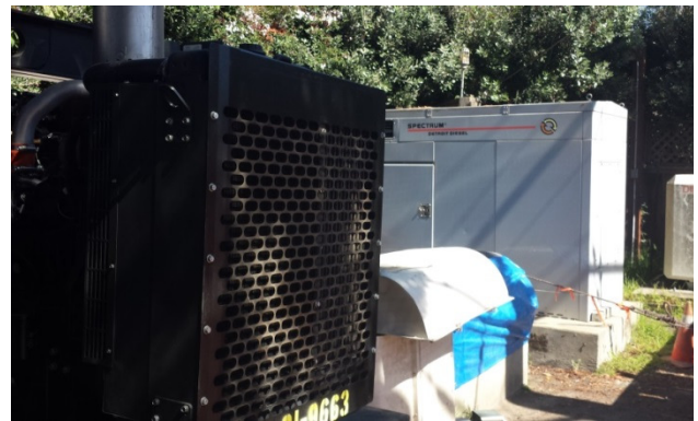
BPUD lift station and backup generators. The building extends 25 feet underground. Credit: Van Belleghem
