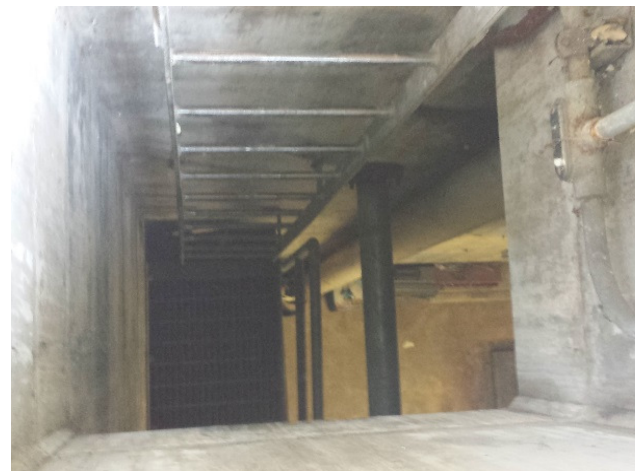
Bolinas Lift Station extends 25 feet below ground. Credit: Van Belleghem
