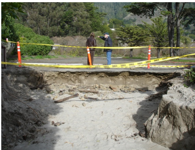
Washed out parking lot, Stinson Beach. Credit: Marin County DPW
