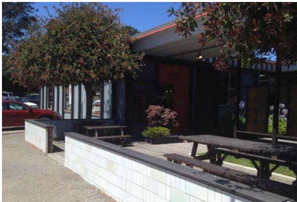
Low-tiered flood wall and gate installed at a commercial building in Marinship. Opening allows for manual insertion of a flood barrier.
