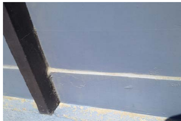
Waterproof paint on bottom few feet of building.
