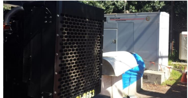
BCPUD lift station and backup generators. The building extends 25 feet underground. Credit: CDA
