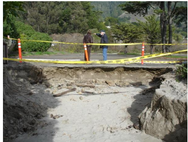
Washed out parking lot, Stinson Beach. Credit: Marin County DPW
