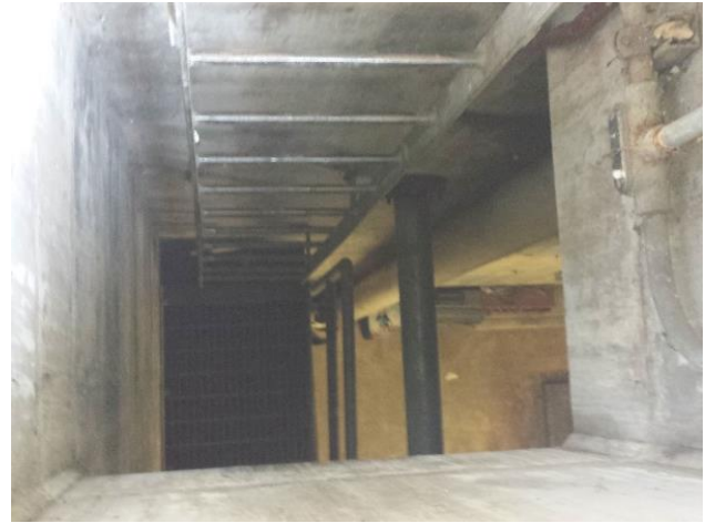
Bolinas Lift Station extends 25 feet below ground. Credit: CDA
