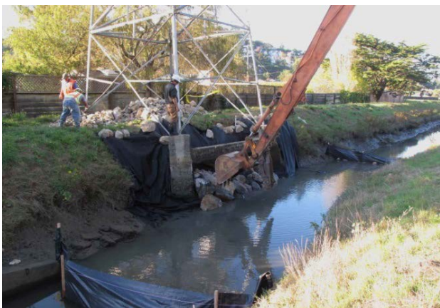
PG&E repair from storm damage in Tamalpais Valley. Credit Marin County DPW
