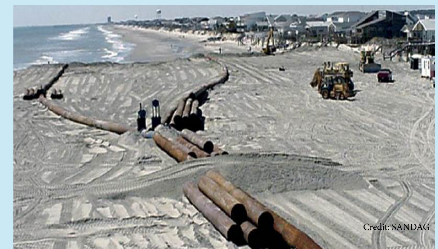
Beach nourishment through hydraulic dredge discharge on beach, spread with land-based construction impact.
