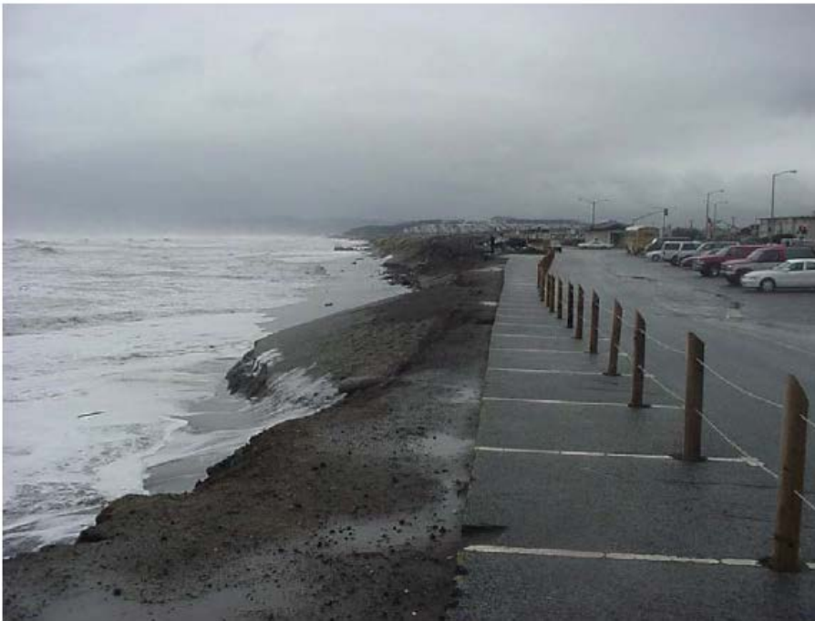
Figure 9: South Ocean Beach: Top: Post construction in 1990s. Bottom: eroded in early 2000s. The wood posts (top photo) were removed by erosion, and were replaced in the parking remaining parking lot (bottom photo). Photographs, Bob Battalio.
