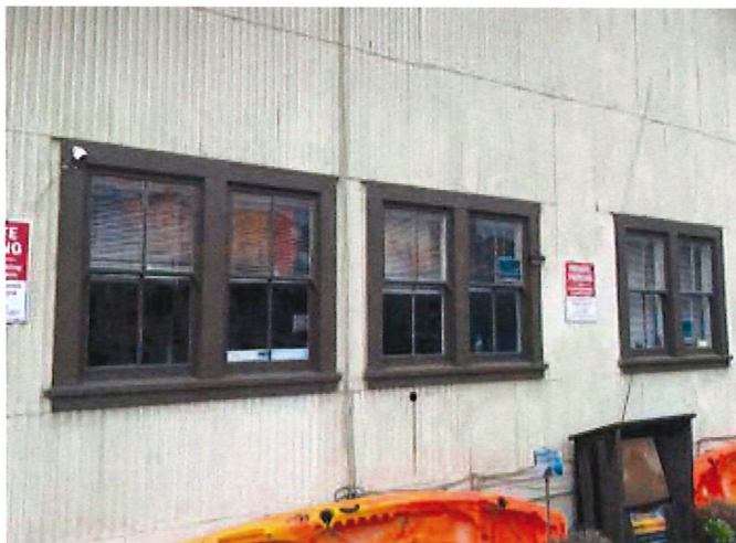
Historic window fabric and placement, January 21, 2024.
