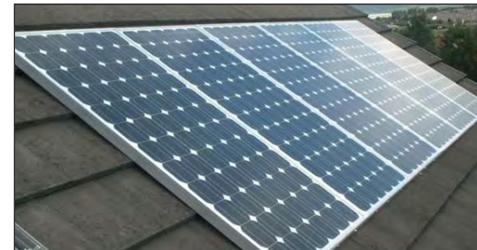
Home solar panels Credit: Marin County Energy Program
