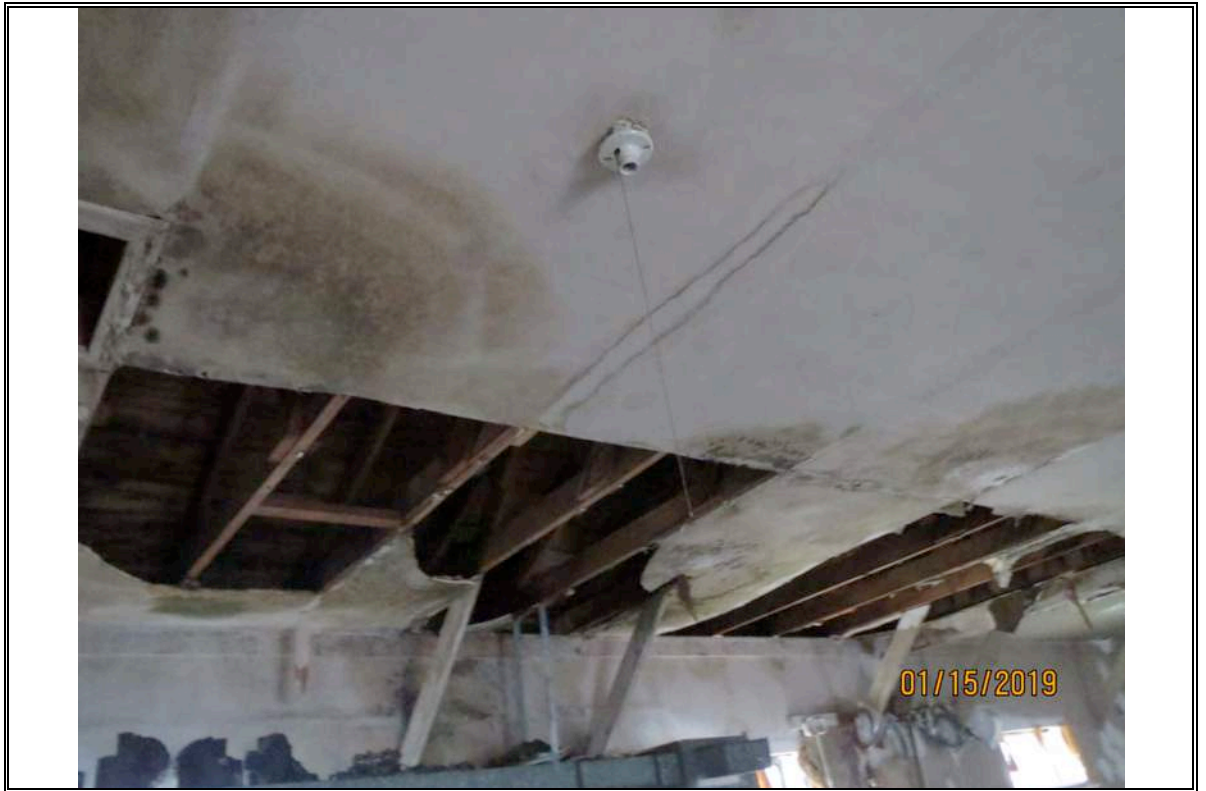
Photograph Number 11: View of the building interior, water damage
