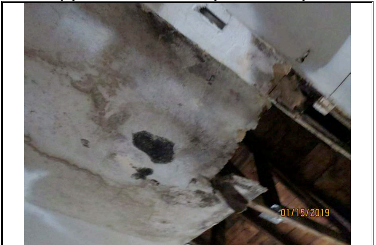
Photograph Number 12: View of the building interior, water damage
