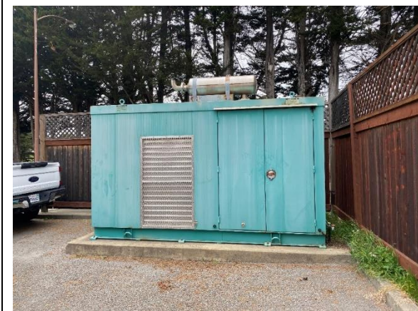
Photo 9: View of diesel generator located next to the Galley Building.
