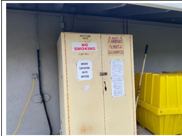
Photo 18: View of chemical storage cabinet located behind the workshop.
