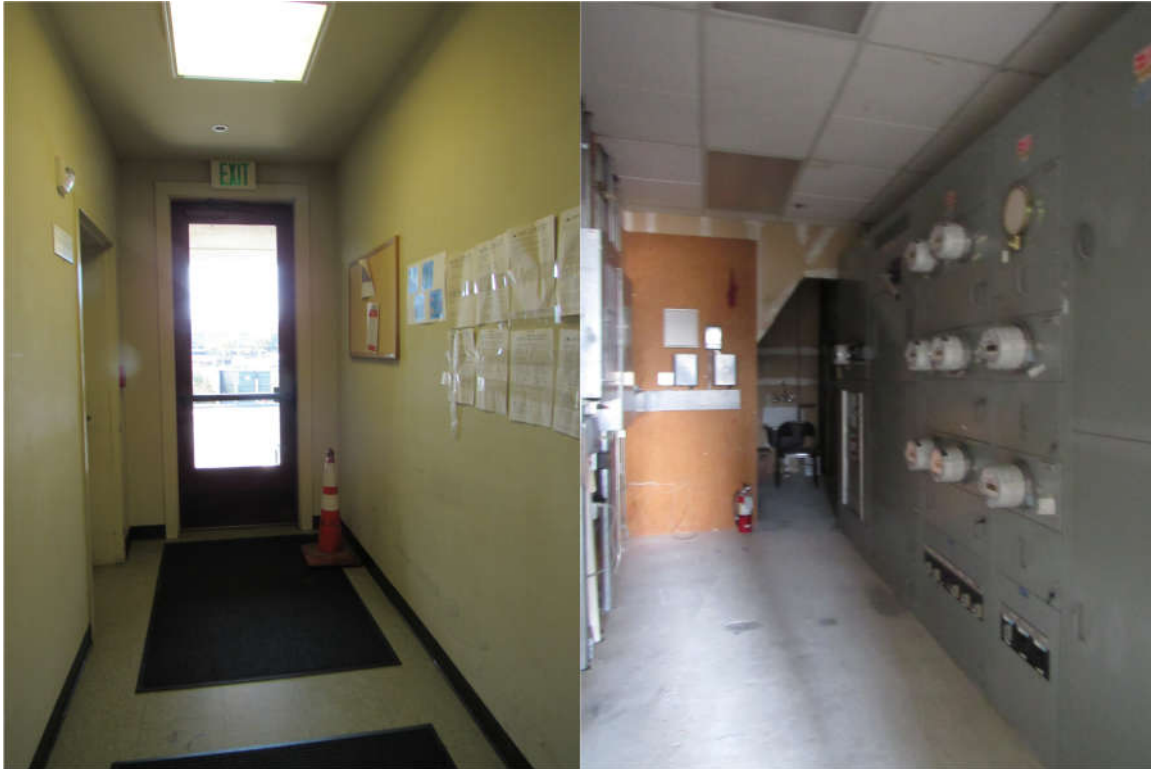
First floor- view to the southwest entry door- electric room
