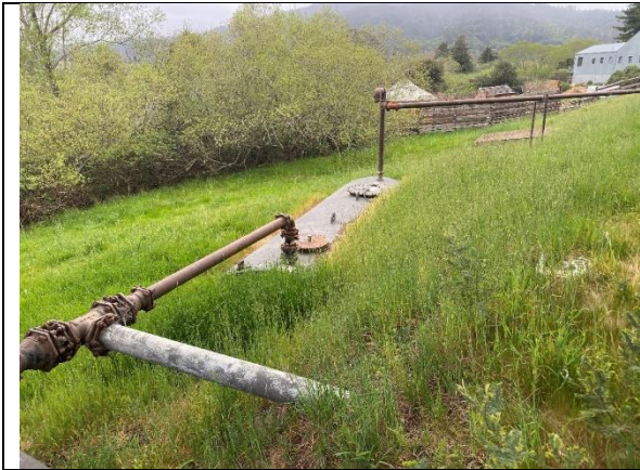
Photo 3: View of partially underground storage tanks near the turn-about off Commodore Webster Drive.
