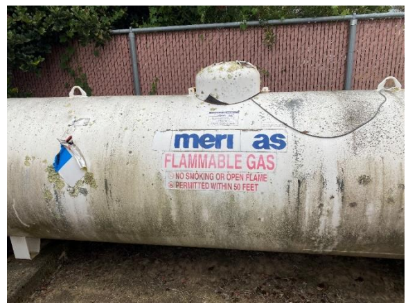
Photo 10: View of above ground propane tank near the Galley Building.
