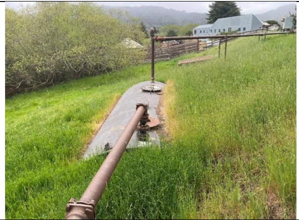
Photo 4: View of partially underground storage tanks near the turn-about off Commodore Webster Drive.
