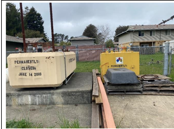
Photo 20: View of two above ground fuel storage tanks located northeast of 100 Commodore Webster Drive.
