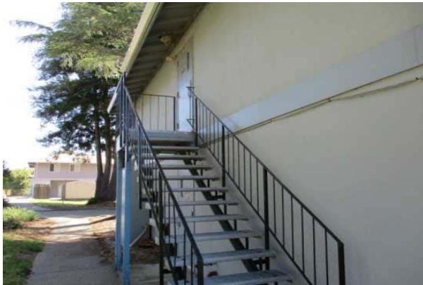
#39: EXTERIOR STAIR RAILS, METAL
