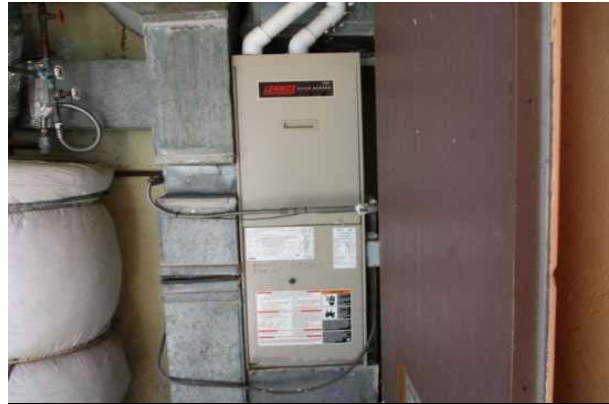
#44: FURNACE, GAS, 101 TO 150 MBH
