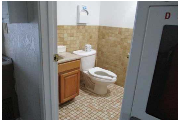
#27: ADA, RESTROOM NEEDS GRAB BARS AND BLOCKING
