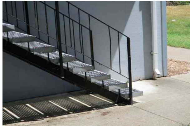
#28: ADA, STAIRS, HANDRAIL EXTENSIONS NEEDED
