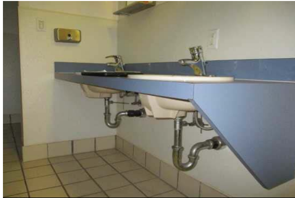
#25: ADA, RESTROOM, LAVATORY PIPE WRAPS
