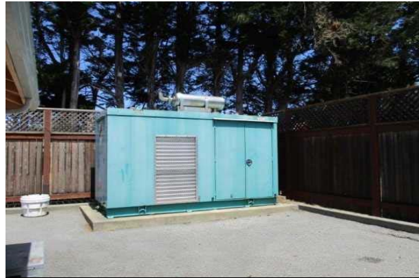
#14: EMERGENCY GENERATOR (COMPLETELY DISCONNECTED)
