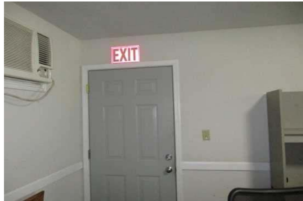
#22: ADA, DOOR, NON COMPLIANT HANDLE HARDWARE
