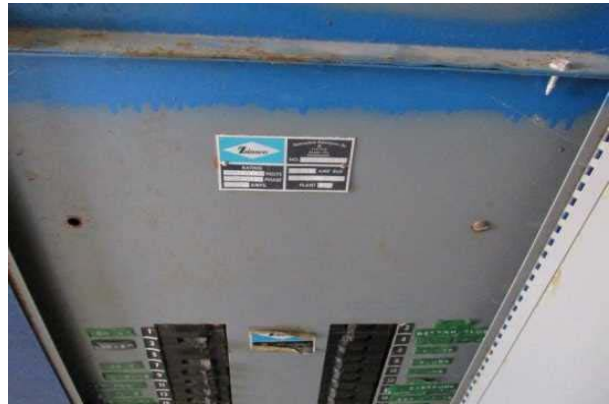
#52: DISTRIBUTION PANEL, 208 Y, 120 V, 400 AMP
