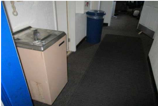
#21: ADA, NON COMPLIANT DRINKING FOUNTAIN
