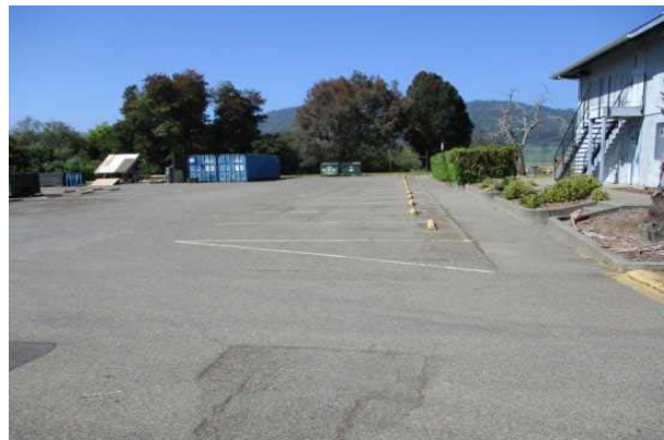
#24: ADA, PARKING, ACCESS AISLE STRIPING NEEDED
