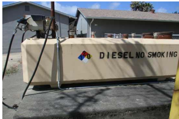
#16: DIESEL FUEL TANK
