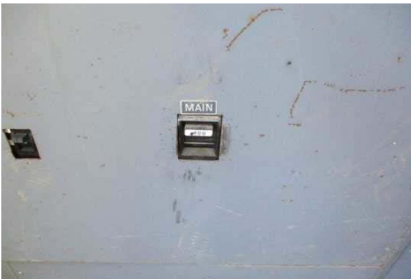
#53: BUILDING/MAIN SWITCHGEAR, 208 Y, 120 V, 400 AMP
