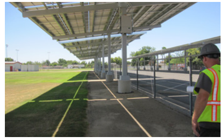
Solar canopy - Rincon Valley USD
