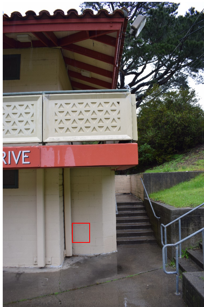
Figure 3: Photograph of the proposed insertion point of the French drain (outlined in red), located at the south end of the primary (west) façade of Building 49, facing east. Courtesy: ICF 2020.
