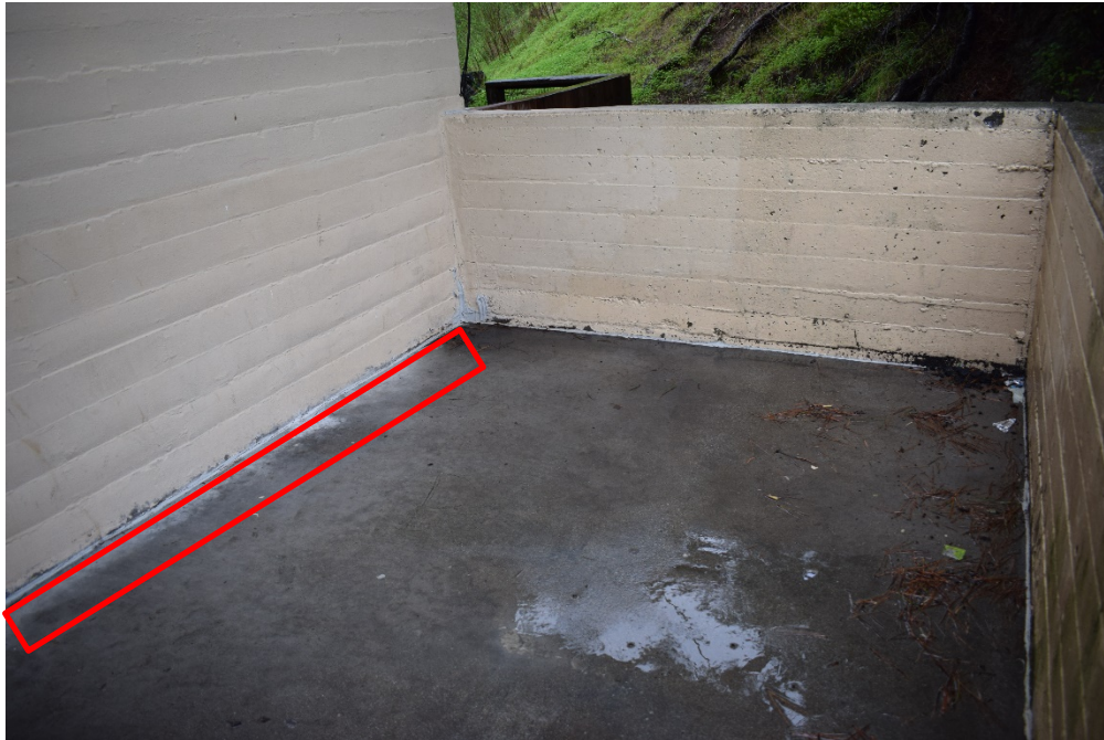
Figure 6: Photograph of the proposed French drain location (outlined in red), would be located within the ground level landing in the south stairway at Building 49. Courtesy: ICF 2020.
