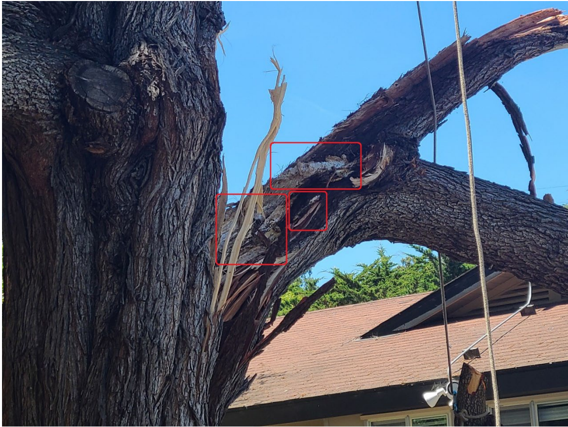
Photo 1 Evidence of white fungal growth in one of the rotted areas of the tree. Source: MHA, 2022. Notations by ICF. 2023.
