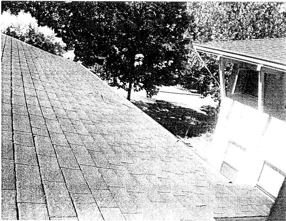
Lump in roof at 5 Frustruck
