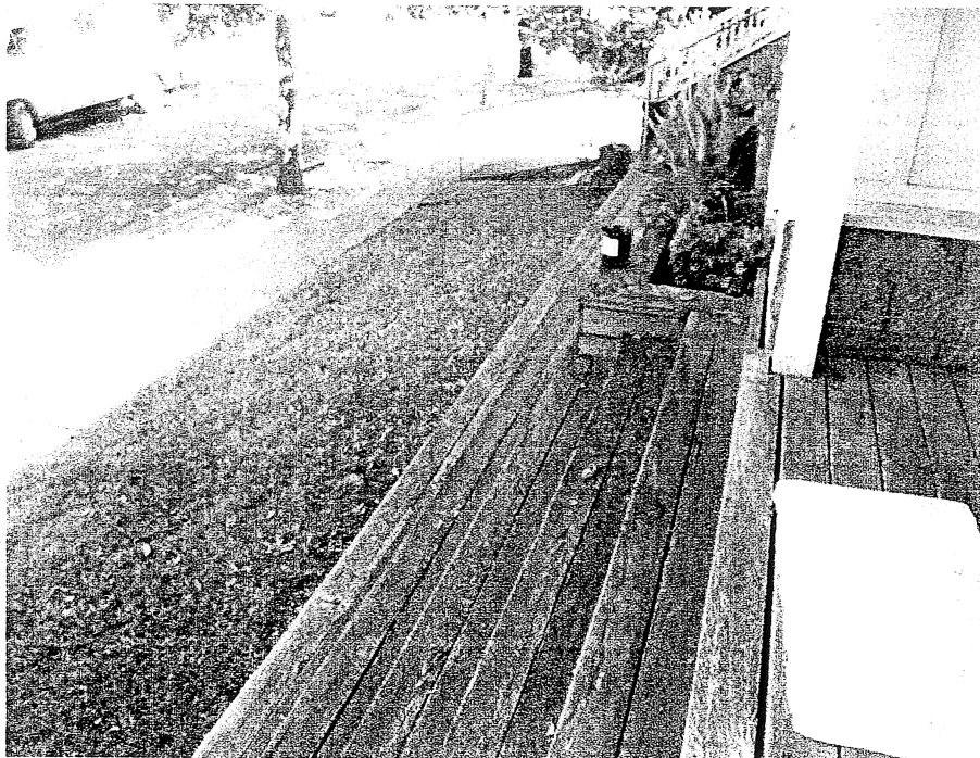
Entry deck boards at 75 Frustruck. Nosing board is very loose.
